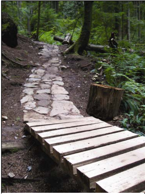
Armoured approach to this TTF increases longevity of the structure, Natural High, Fromme Mountain.
