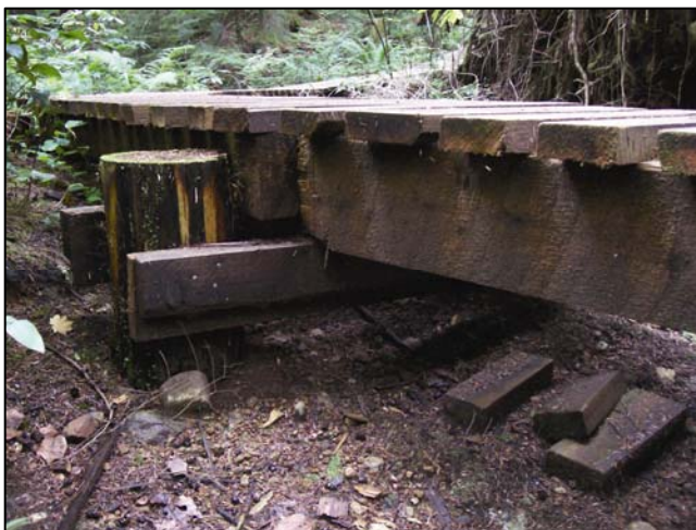
Bridge stringers elevated above ground to reduce potential for rot, Natural High, Fromme Mountain.
