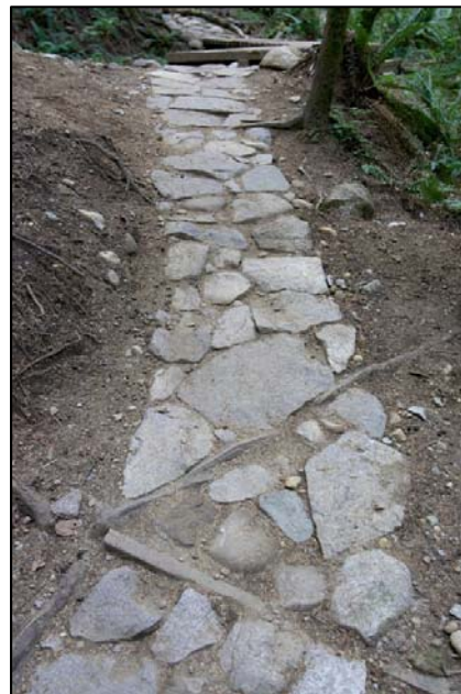
Figure 4: Successful rock armouring techniques include favouring angular stone where available over rounded stones.
